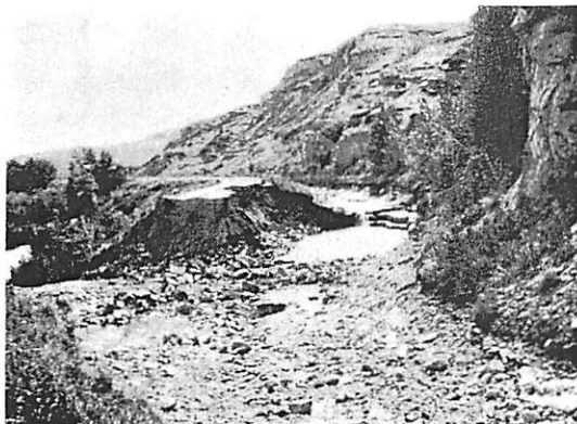
LEFT: One of the major breaks on the main Two Medicine canal. This photo was taken shortly after the flood of June 8, 1964.
